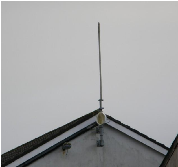
Transmitter Site Photo
